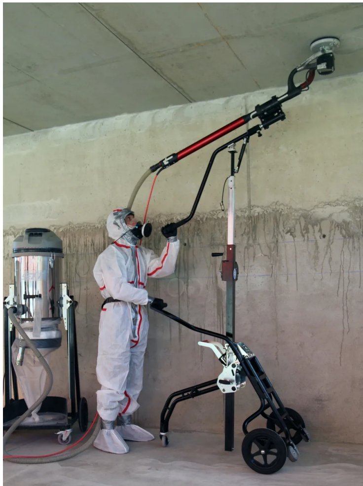
Ceiling sanding with Sept Tools system – up to 8 hours of continuous work without fatigue
